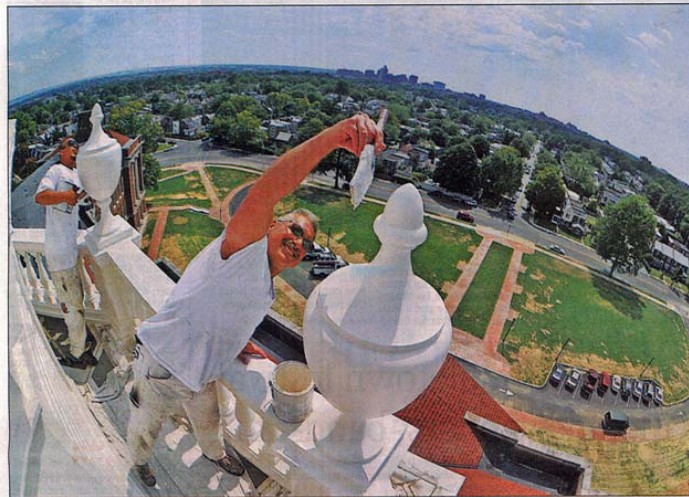
The News Journal/FRED COMEGYS Painters Frank Kaminski (foreground), and Julio Santiago put finishing touches Thursday on the cupola of the P.S. du Pont Elementary School, or 'The Palace,' as it was known to students in the 1930s and 1940s. "It was made by true craftsmen, and I'm proud to renovate this building," said Michael Petka, project manager for Bancroft Construction Co. of Wilmington, the primary contractor. The school's $44 million renovation is one of the most expensive in Delaware history. On the horizon is the Wilmington skyline. See story on B3.
